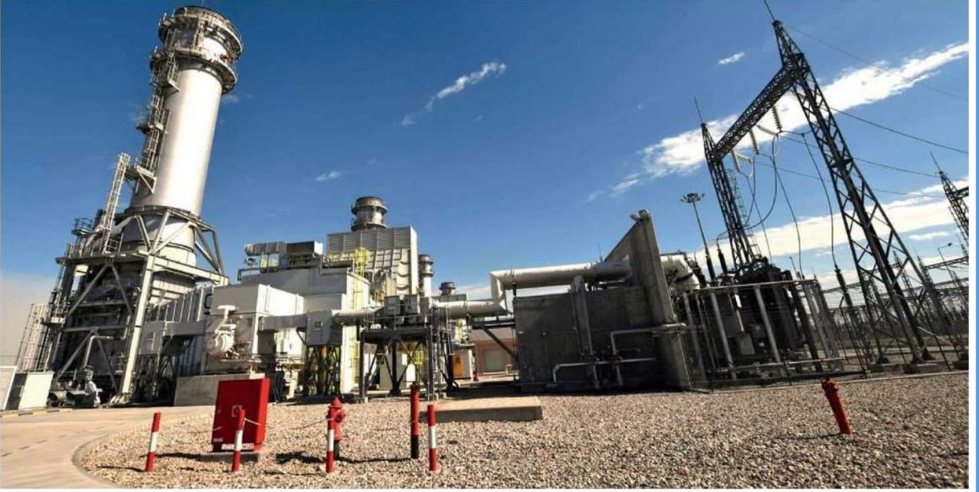
This undated file photo shows a power plant near Iraq's Nasiriyah region along the banks of the Euphrates River.
